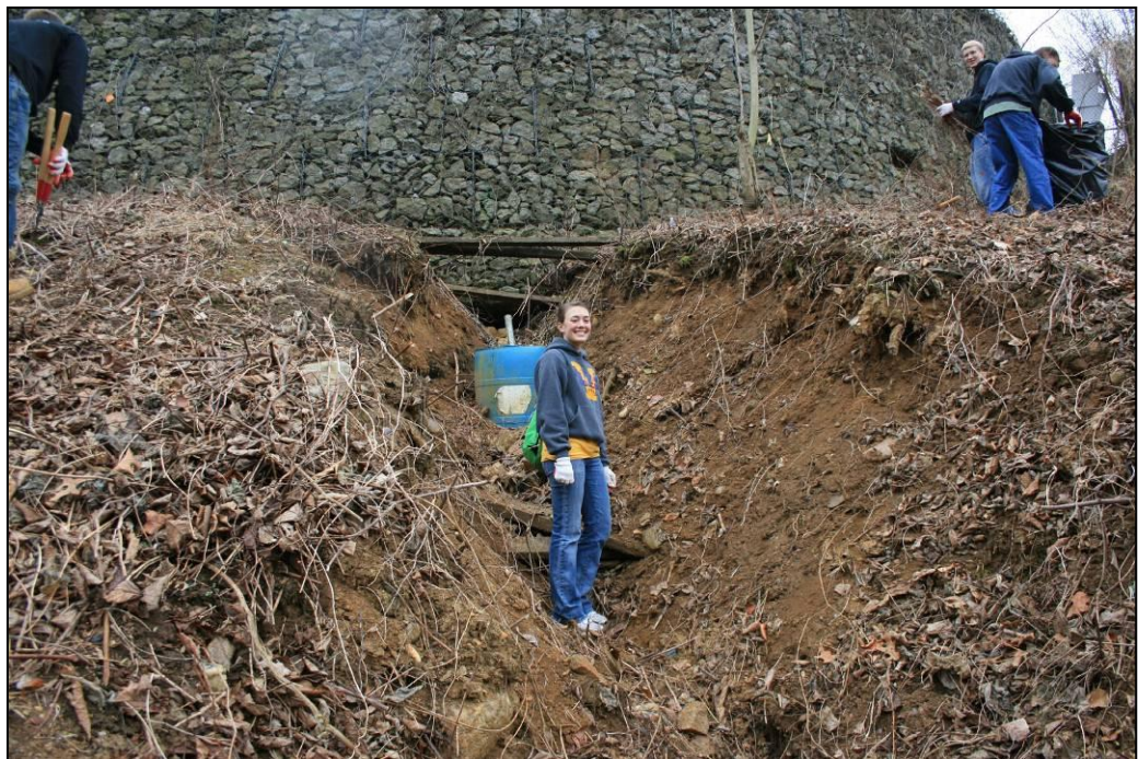
Fig. 42: A Catholic University student at a March 2009 clean-up stands in the larger of two North Slope gullies, which were created by gardeners diverting water from the gabion wall to irrigate their crops.
